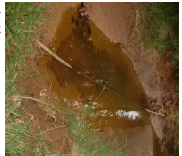
Pictured is a standing pool of flood water where the in-fill of a trench, dug to lay cable for electrical services to the Glenwood Village 2 development, has been washed away.
