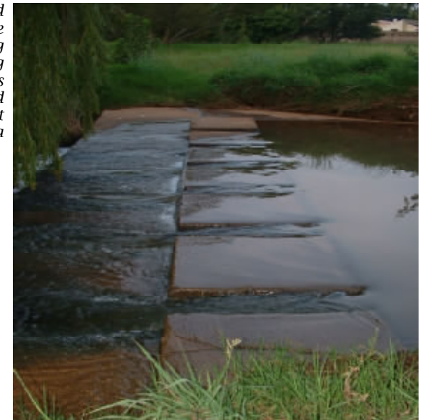
Pictured is the ford south of the Alcade Road gate showing the river overtopping the stepping stones after heavy rain and hampering east-west access in the Moreleta Reserve.
